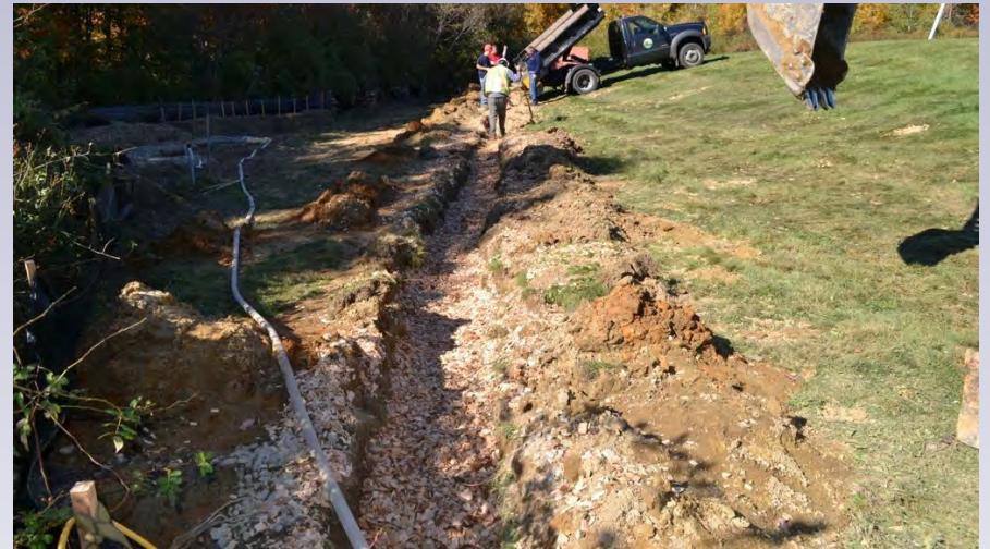
RCCD implementing the first installation in New Hampshire of a new innovative technology to reduce nitrogen from septic system leachate. Brentwood, NH.
